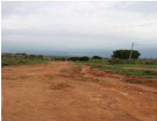
Figure 7: Condition of Gravel Roads
