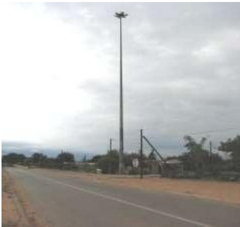
Figure 3: High Mast Lighting in Sebayeng
