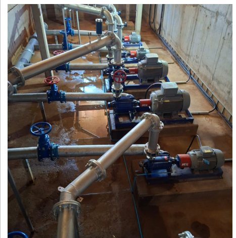
Newly installed pumps at Molepo Water Treatment Plant
