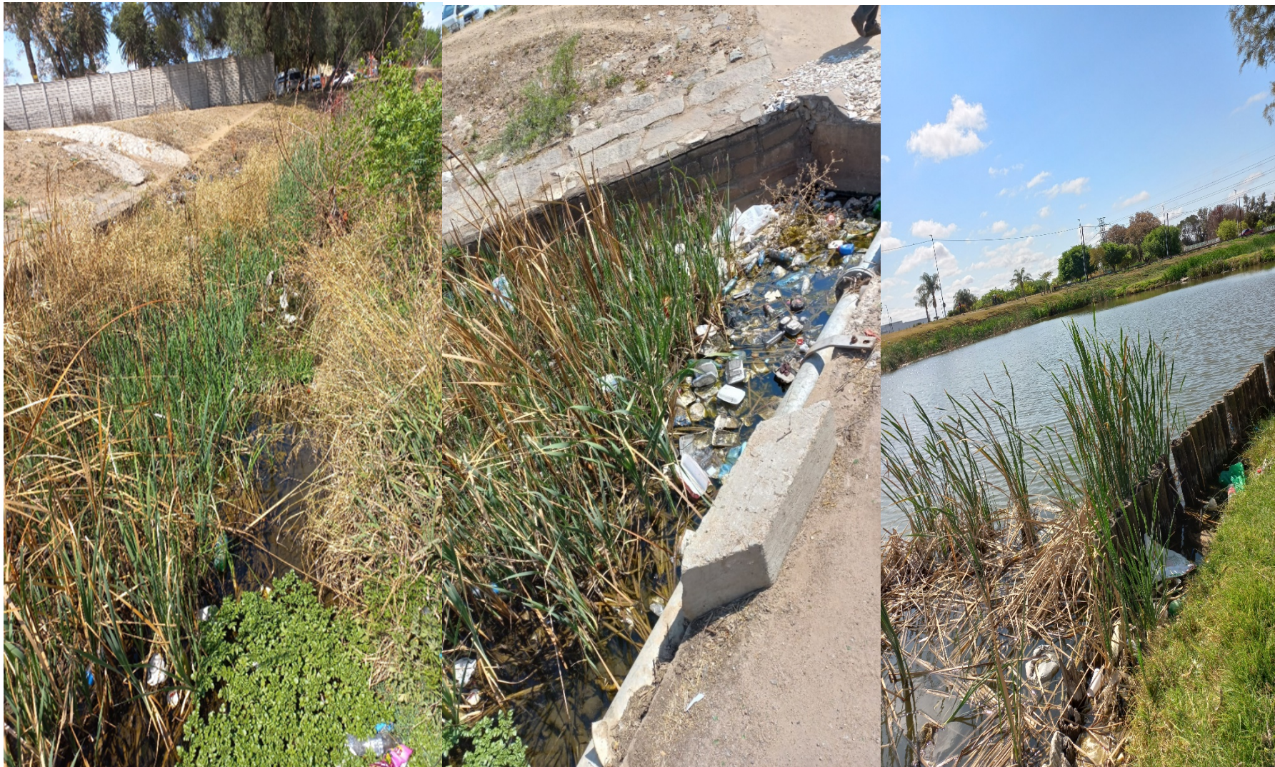
Diagram 190: Overgrown vegetation and litter noted in the drainage lines and stormwater infrastructure.
