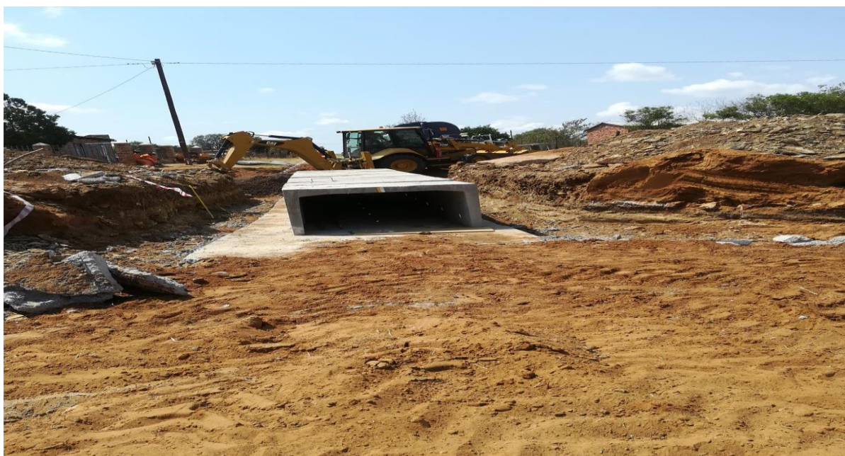
Stormwater management infrastructure as Ga-Semenya
