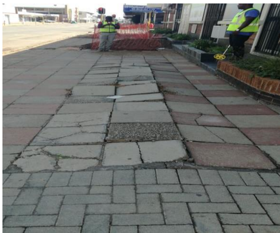
Section heaving after pipe jacking
