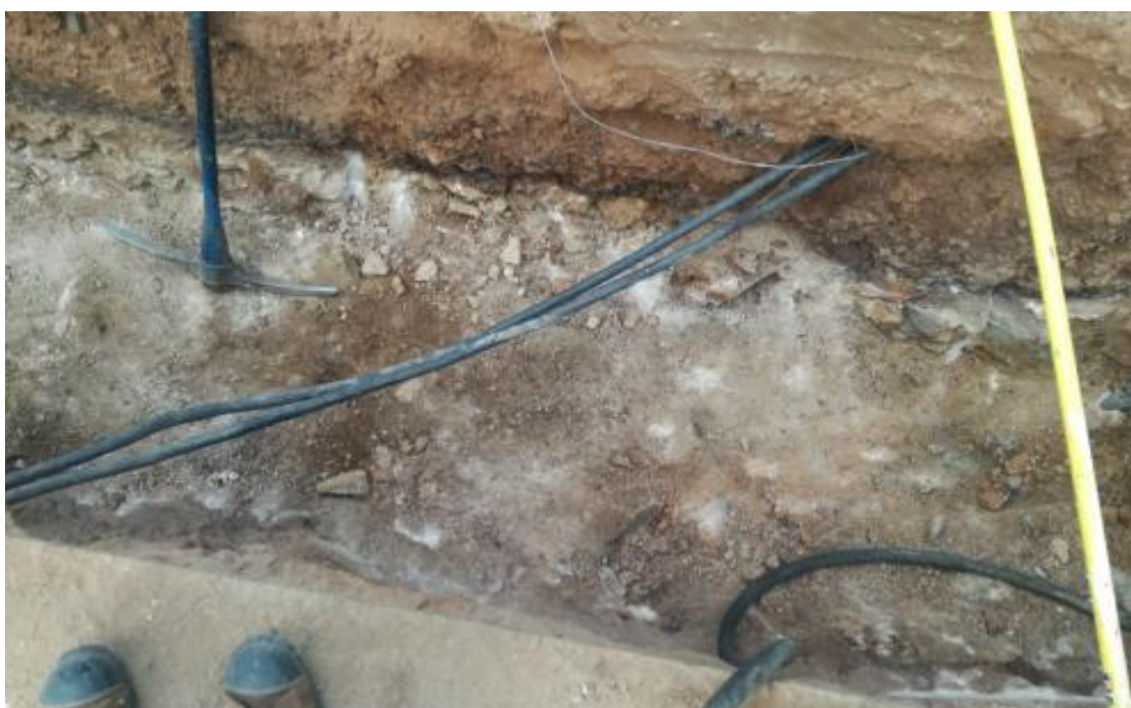
Hard rock and underground services pose a challenge in the CBD and requires open excavations.
