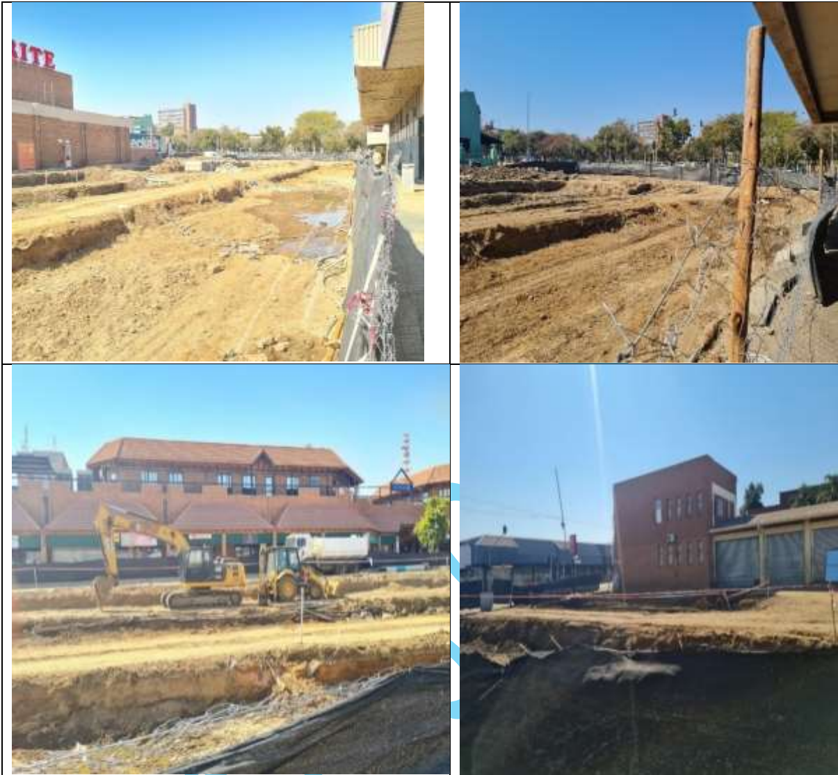
Construction of the Leeto la bus Station on General Joubert Street (10 August 2021)
