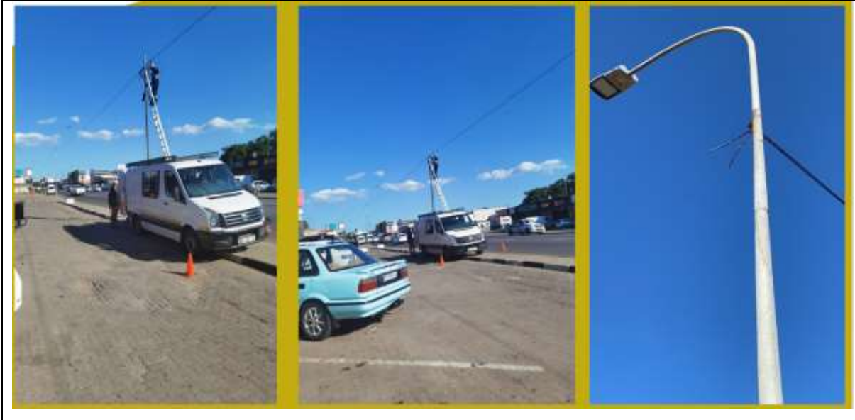
Source: PLK Information Communications and Technology (ICT) SBU (2021)
