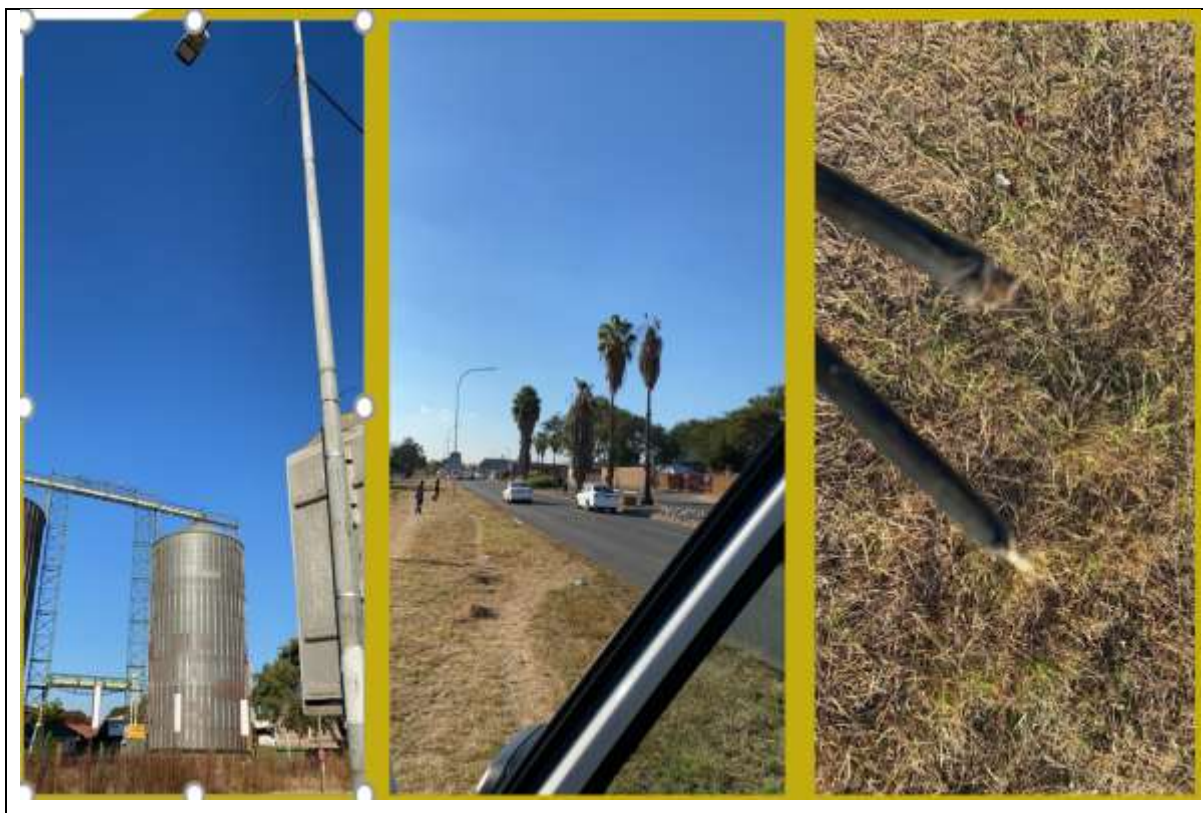
Figure: Damage and repair process of fibre connection.
