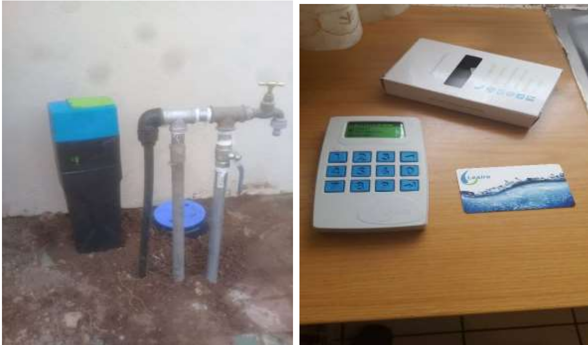
Prepaid Water Smart Metering
