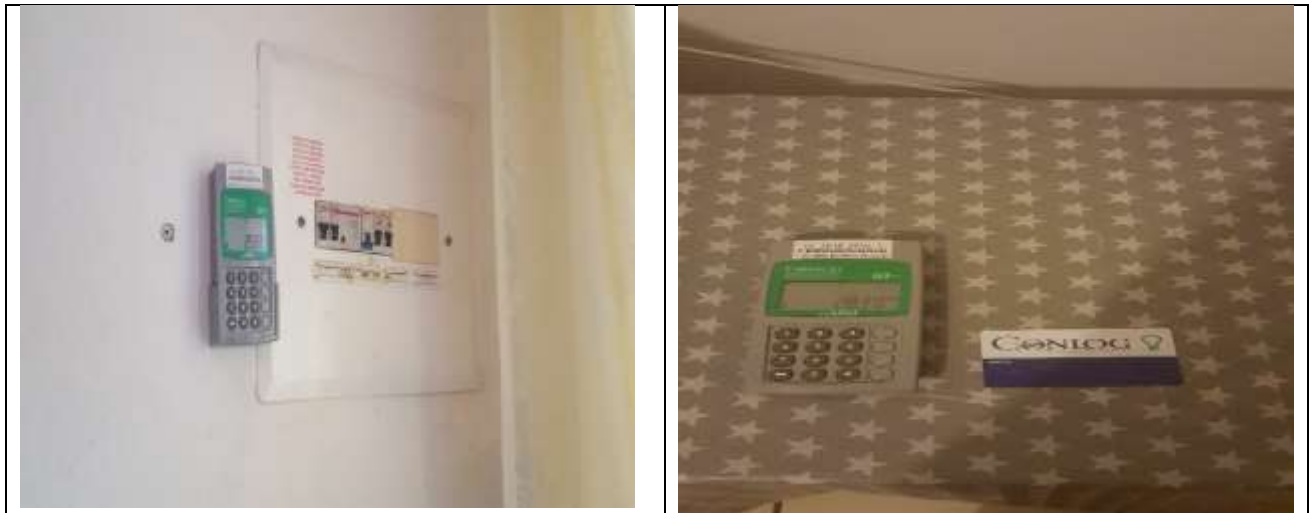
Pre-Paid Electricity Meters
